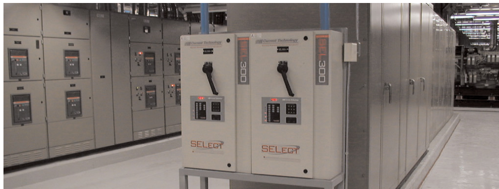
Two Select® SL 300s protect Triara's service entrance and several TransGuard® TG100s protect downstream equipment.
