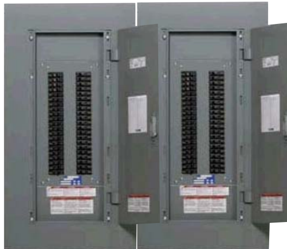
Two 42 Circuit Panelboards
